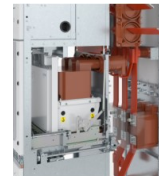
Current and voltage transformers located in the bus riser.
