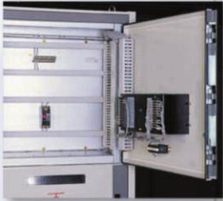
Low Voltage Compartment
